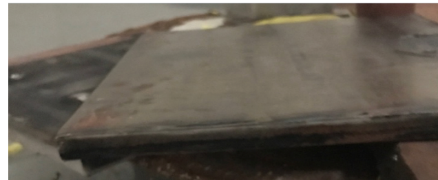
Figure 18 Flat 1" thick steel plate with paint and corrosion
